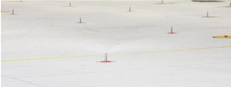
Figure 1 – Pop-Up Foam Sprinklers Operational
