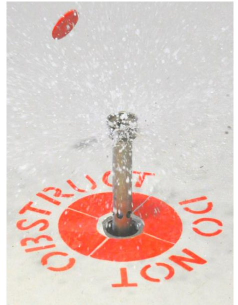
Figure 3 – Pop-Up Foam Sprinkler Operational
