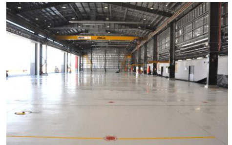
Figure 6 – Typically Discreet installation of ARCHER Pop-Up Foam Sprinklers
