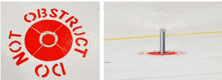
Figure 2 A & B – Pop-Up Foam Sprinkler on Standby and Operational
