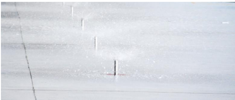
Figure 4 – Pop-Up Foam Sprinklers in Action
